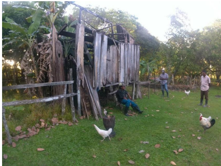
Photo 7 Picture depicting the vulnerability of local infrastructure to storms that are increasing in frequency and intensity.
